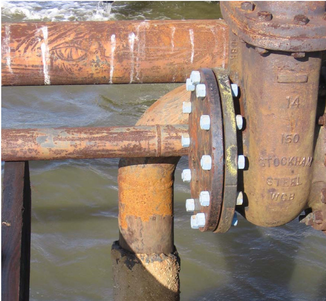
Figure 14. Beginning of the gas sales pipeline (vertical pipe entering water) at the Gulfport sales platform in the West Cote Blanche Bay oil field. The pipeline was ruptured by the Athena 106 's aft spud in an east-west section near the Gulfport platform. The pipe's concrete coating is visible above the waterline.
