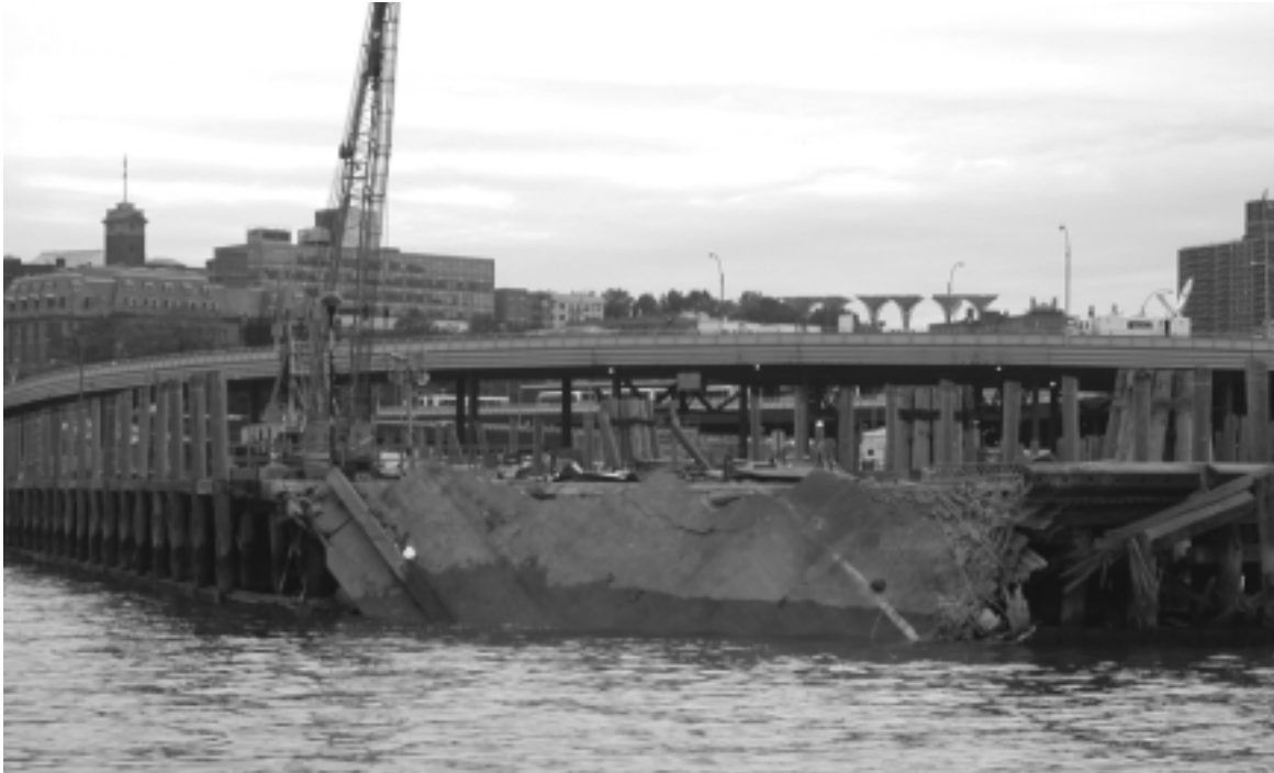
Figure 4. View of damage to maintenance pier caused by Andrew J. Barberi .
